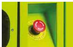
Niche for external emergency push-button
