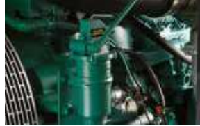
Lube oil drain pump
